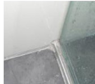
Area of Leak
