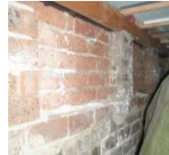
Efflorescence to Wall
