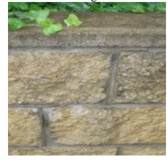
Area of Cracking
