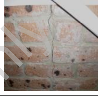
Area of Cracking
