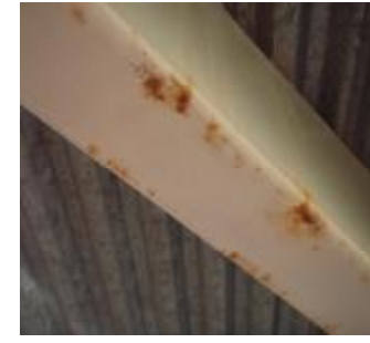
Surface Rust to Beam
