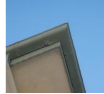
Leaks to Gutter
