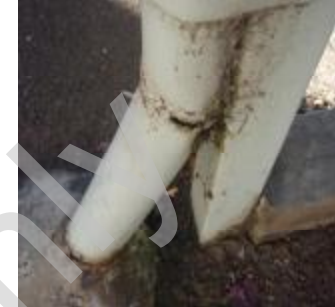
Leaks to Joins
