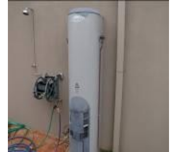
Hot Water Unit
