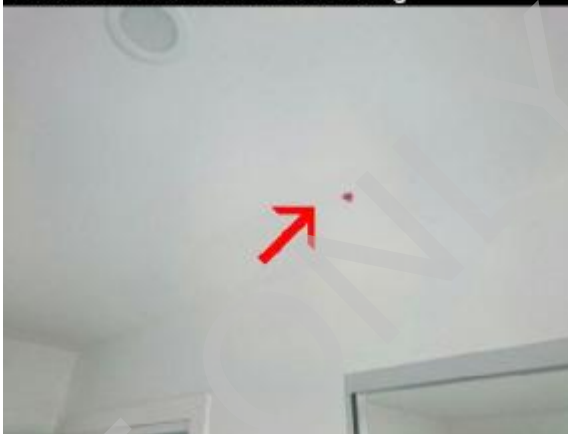
Water stain to bedroom four ceiling
