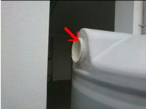
Missing overflow pipe to tank
