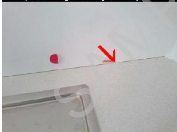
Inadequate sealing to laundry benchtop
