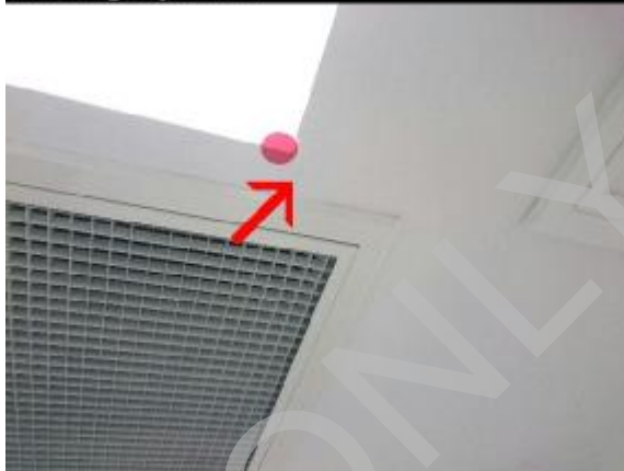
Cracking to join hall
