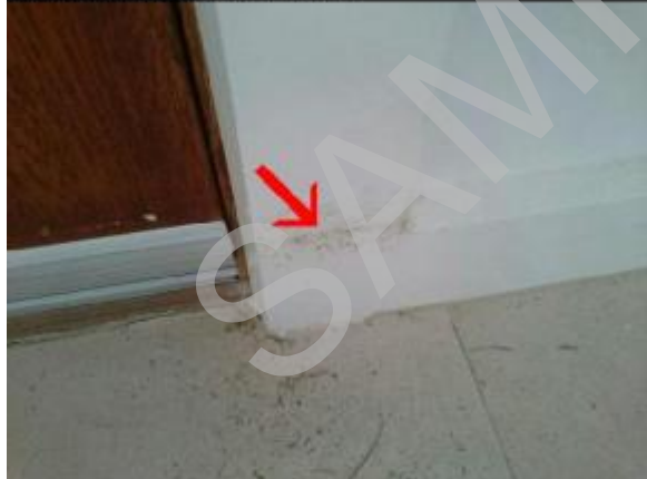
Staining to entry architrave
