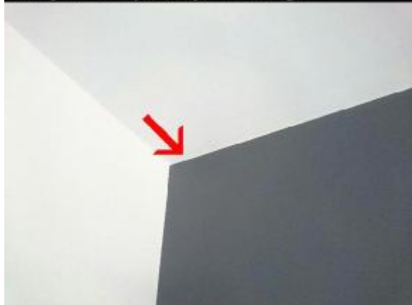
Poorly finished plaster join to lounge
