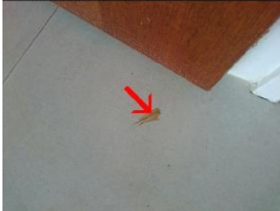
Staining to floor of lounge
