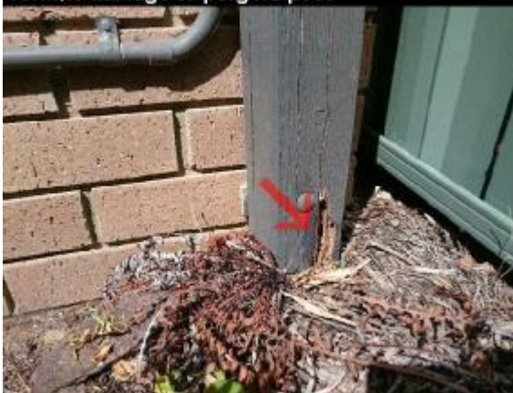
Termite damage to pergola post
