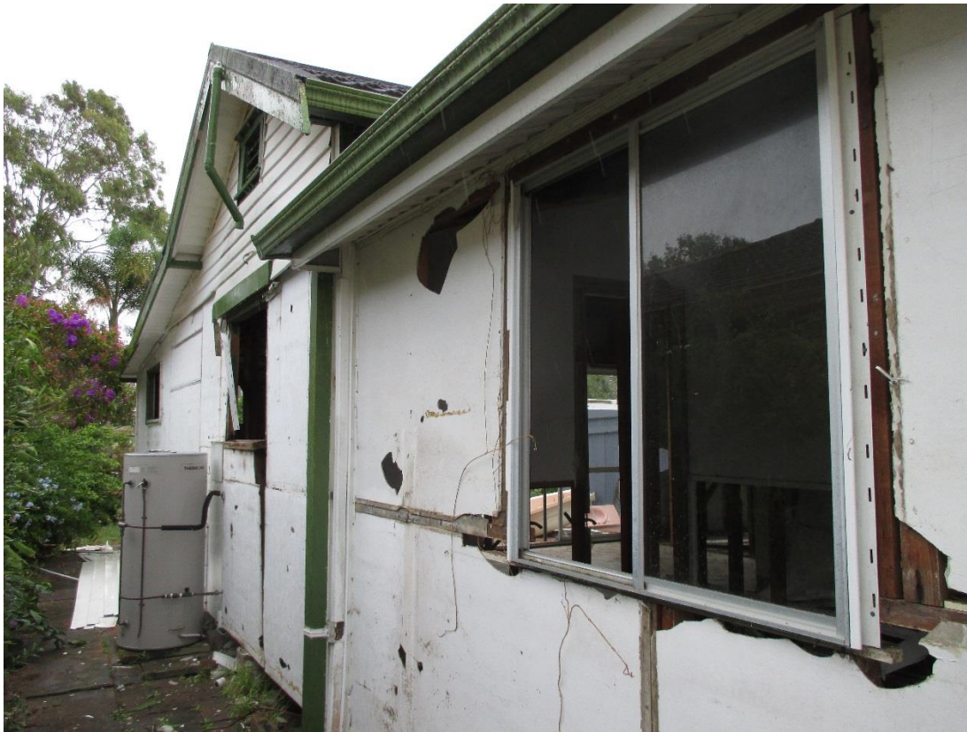
Figure 1: Damage caused to asbestos sheeting when removing connecting strips
