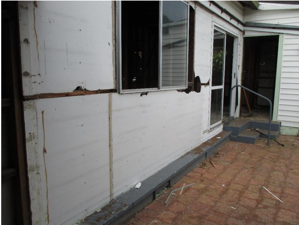
Figure 3: Damage to ACM sheeting in preparation for cladding
